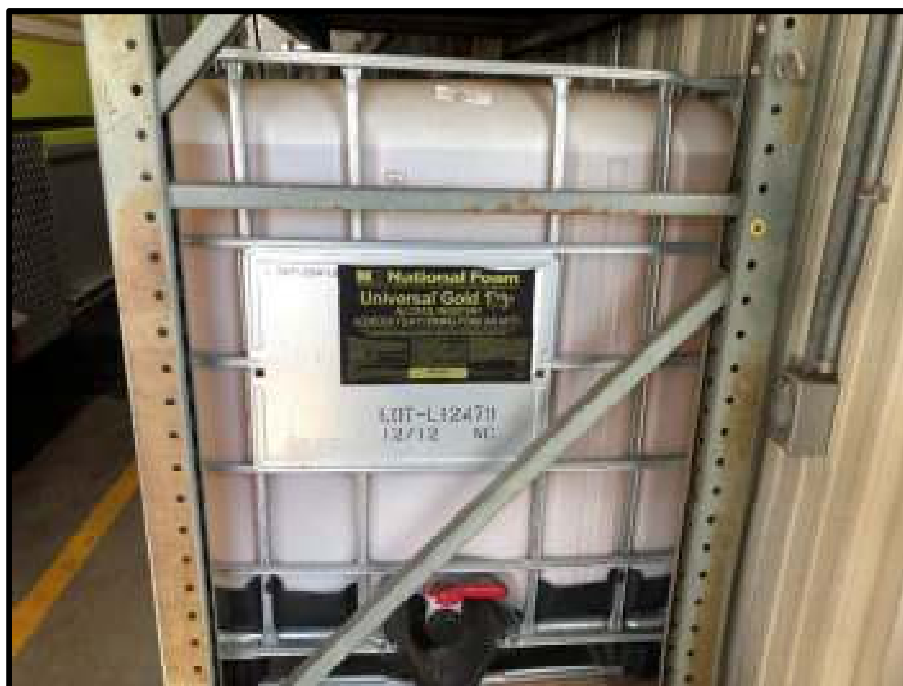
Photograph 7 – View of one of the 660 gallon AFFF tanks within the A.R.F.F.
