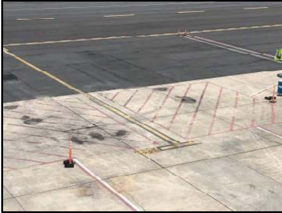
Photograph 5 – View of stained pavement on the apron airside of the terminal building, facing east.
