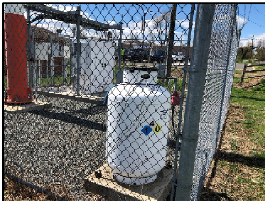
Photograph 8 – View of the propane tank located near the parking lots in the West Area.
